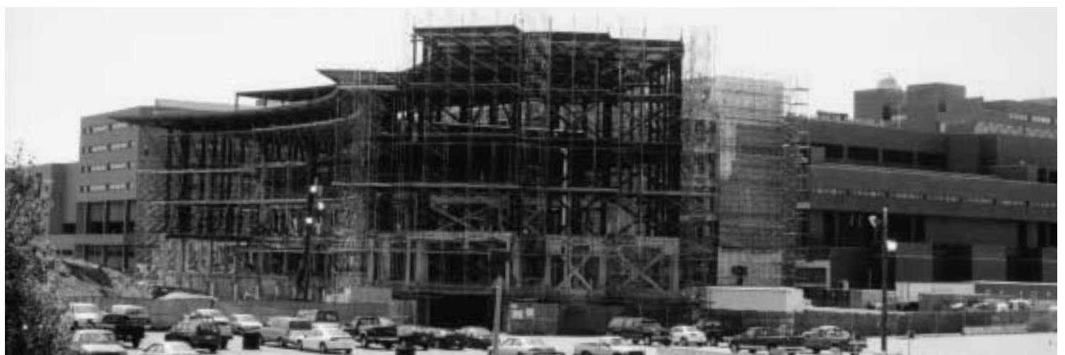
The 331,000 square foot Campus Center will face Boston Harbor and serve as the new front door to the campus.
